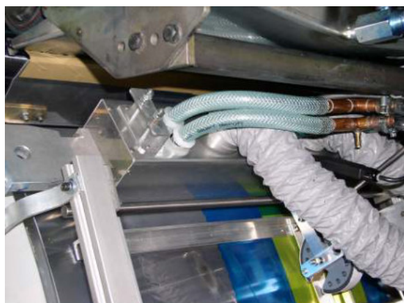
Figure 1: Drying system between the presses.
